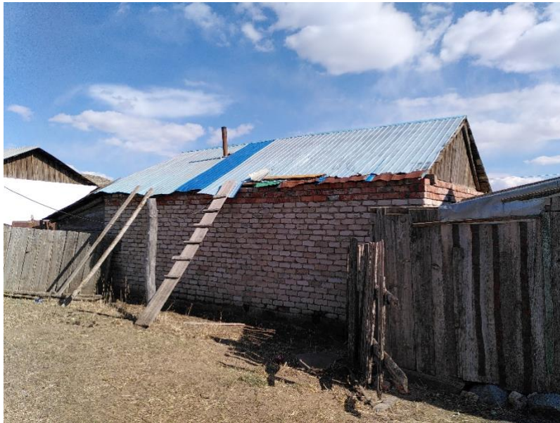
Example of a poorly sealed roof (lack of sealing for the chimney and damaged roof sheets).
