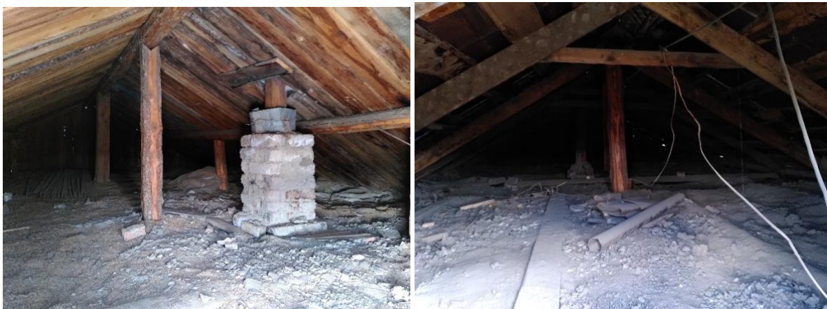
Examples of poor roof structures. On the left, big ridge beam and plank rafters. On the right, structure with poor quality collar ties
