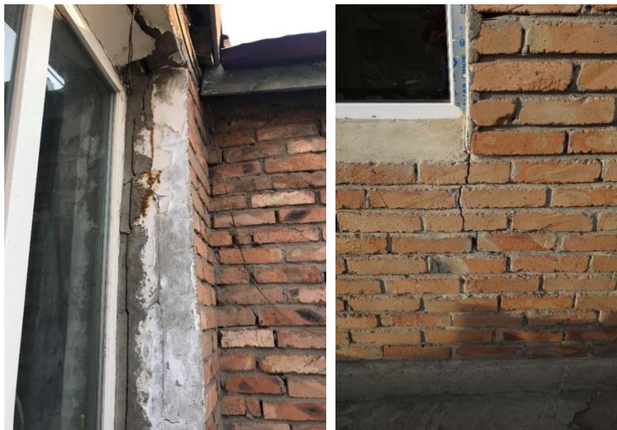
Examples of damages caused by humidity retainment in mixed wall.
